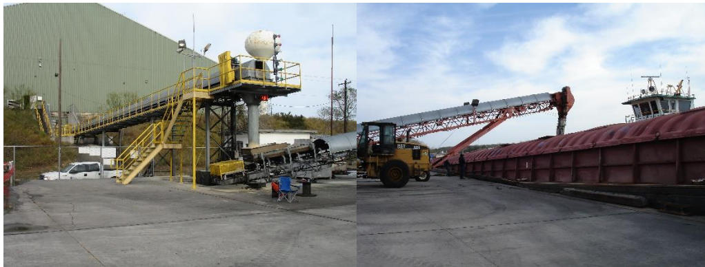
Figure 13 Fixed Conveyor Transfer Unit on Pier, Barge Loading Conveyor
