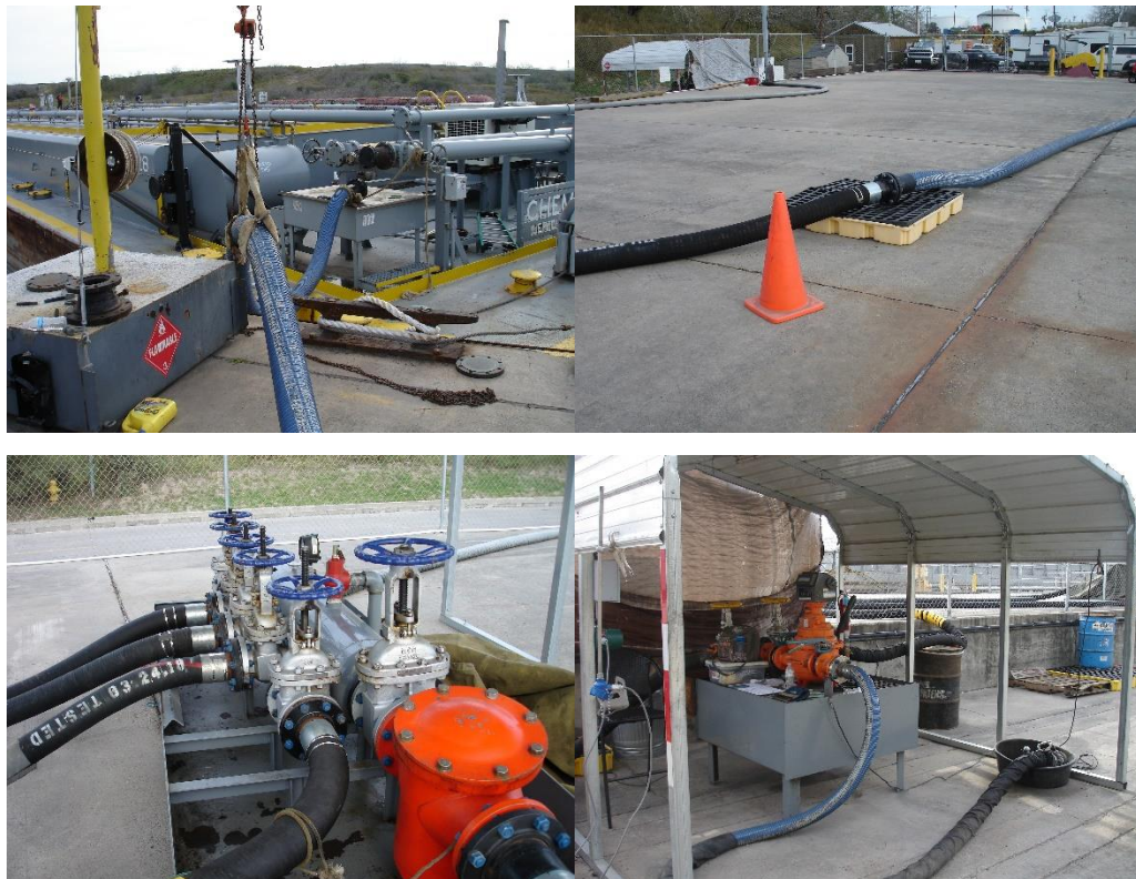
Figure 15 Barge Manifold (Top Left), Pollution Control Tray (Top Right), Truck Distribution Manifold (Bottom Left), Truck Loading Manifold (Bottom Right).
